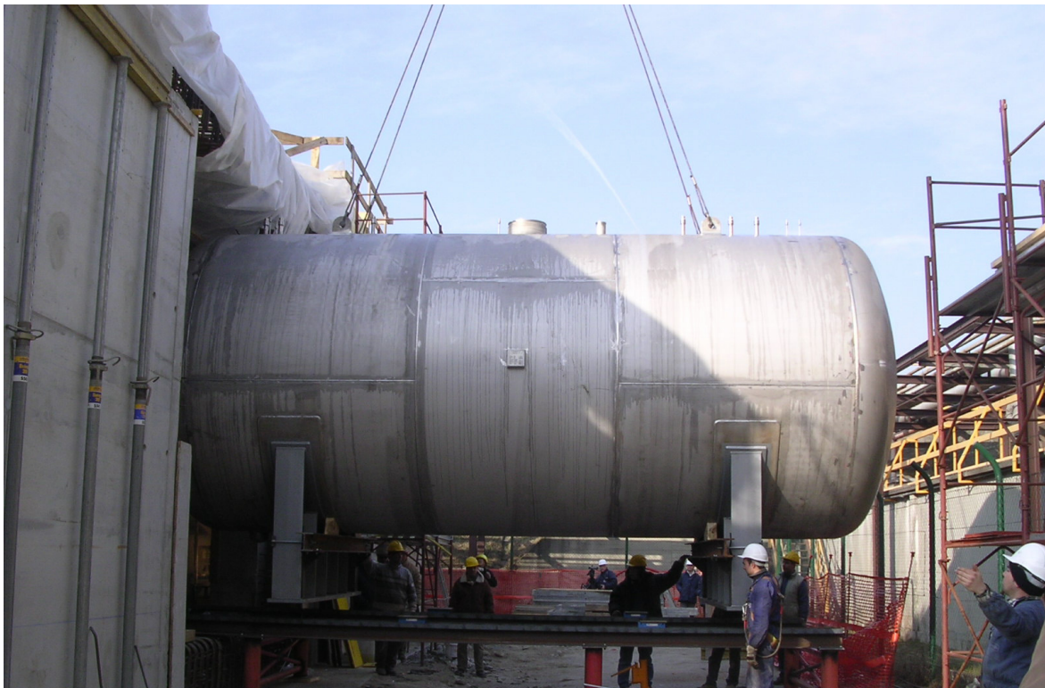
Figure 5: EUREX – One of the tanks of the new storage facility for High level Liquid Waste under construction
