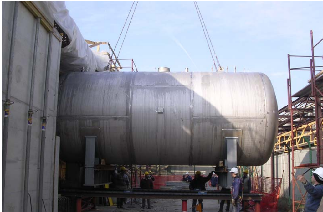
Figure 6: EUREX – One of the tanks of the new storage facility for High level Liquid Waste during the construction
